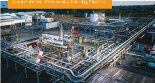
Uquo Central Processing Facility, Nigeria
