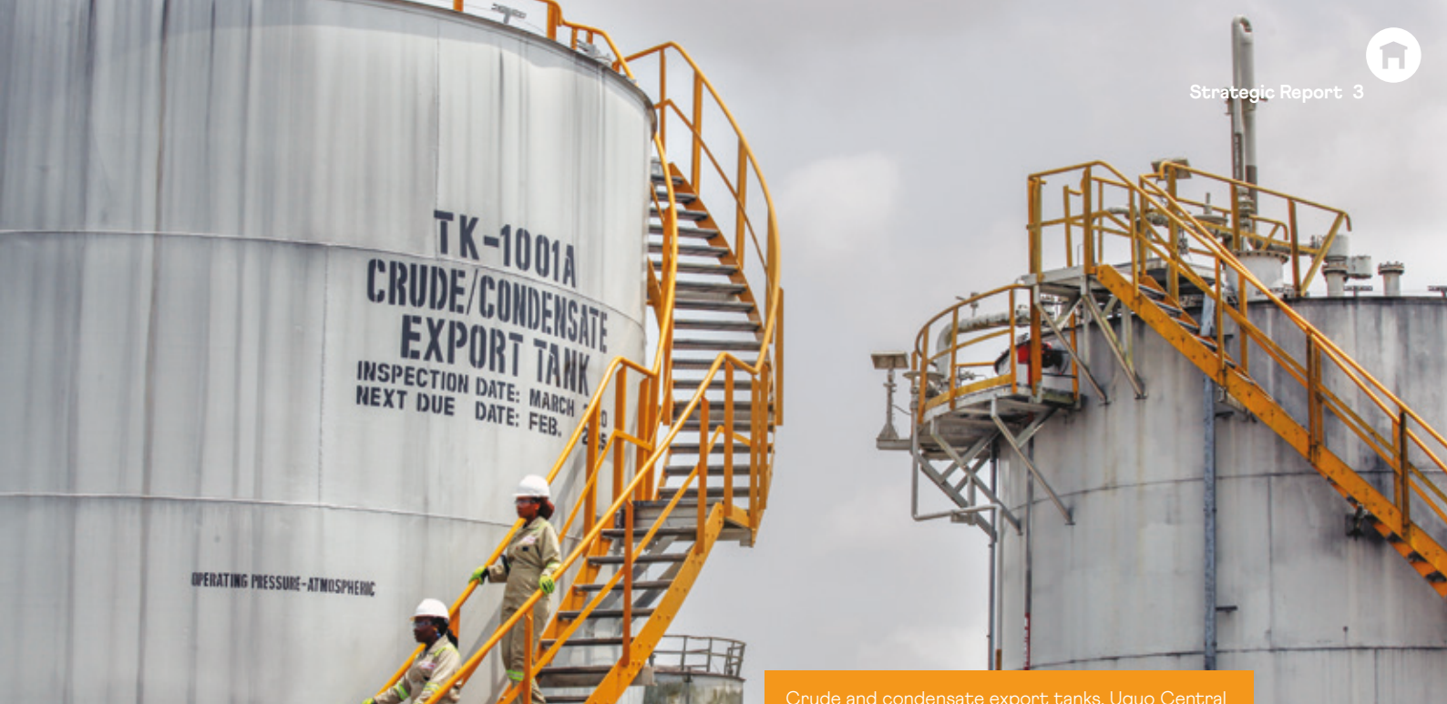
Crude and condensate export tanks, Uquo Central Processing Facility, Nigeria
