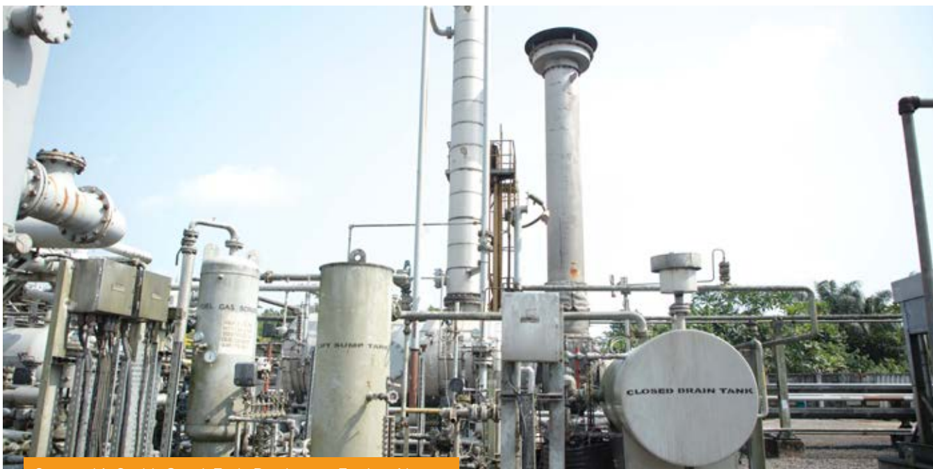
Savannah's Stubb Creek Early Production Facility, Nigeria
