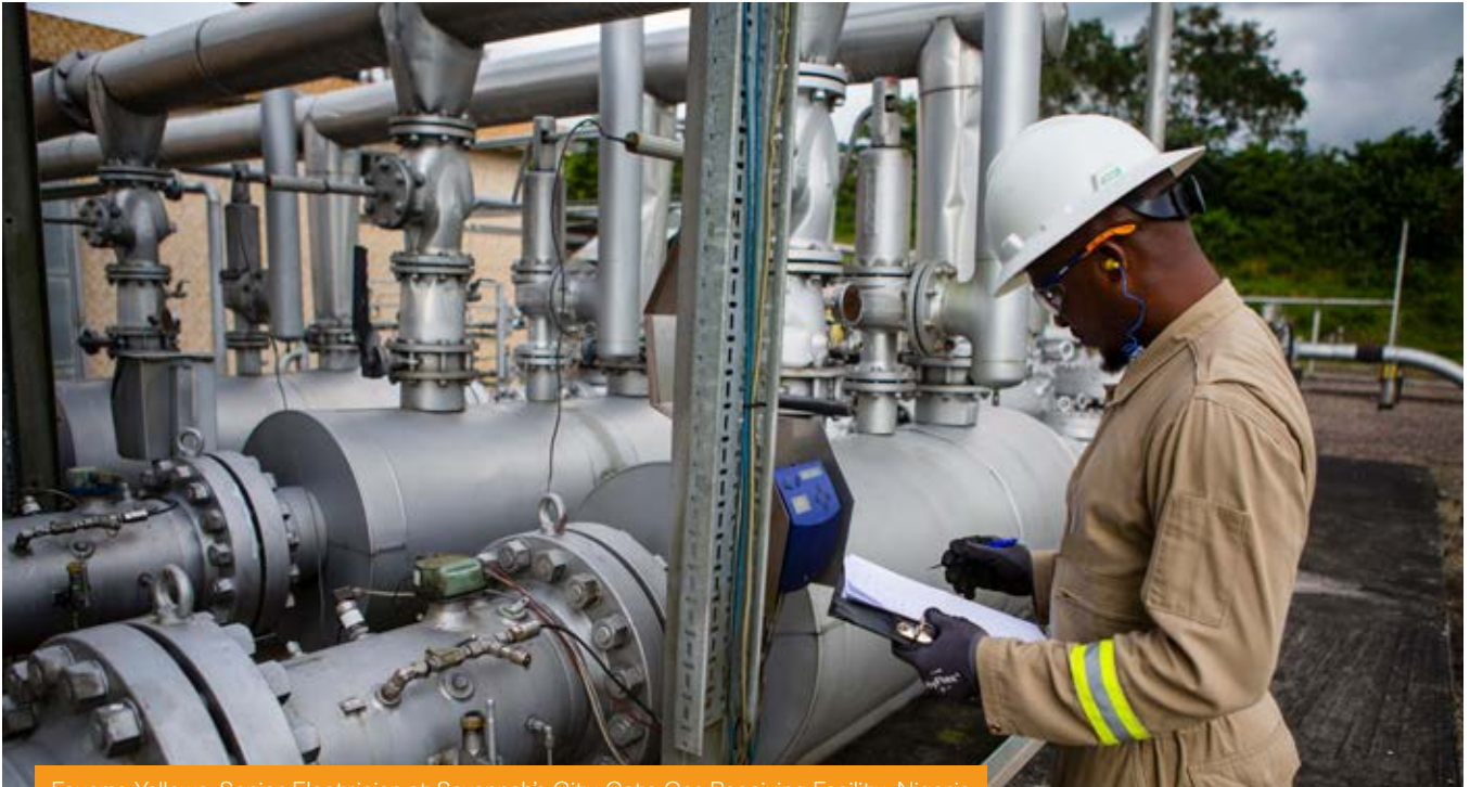
Fayama Yellowe, Senior Electrician at Savannah's City Gate Gas Receiving Facility, Nigeria
