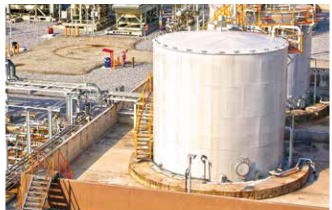
Uquo gas processing facilities
