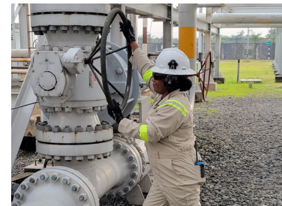
Rosiline Ini-Okor (Field Operator) operating a valve at the Uquo production facility in Nigeria.
